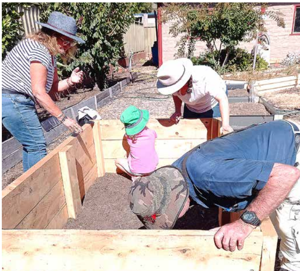
Members of the wicking bed team begin assembling the layered structure of growth materials in the new wicking bed.
