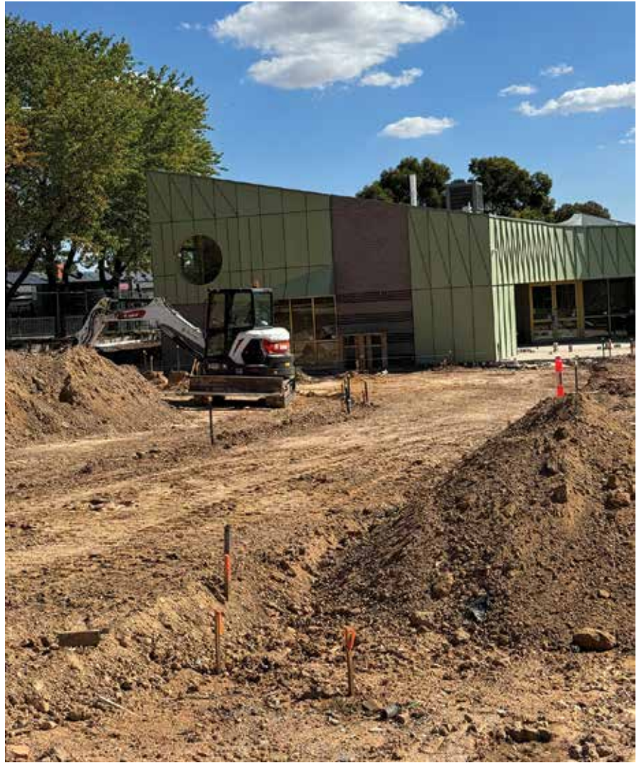
As the term came to an end, the new Technology wing was getting its final touches inside and landscaping had begun. When staff and students return to school on 15 April, they hope to see some BIG changes with the landscaping. Hopefully the college can get to move into this building around week two or three of the new term.
