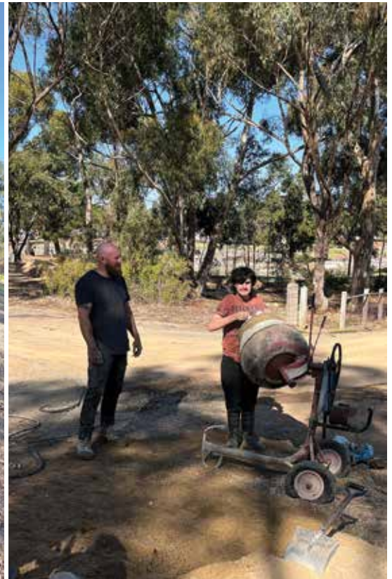
Grant watches over Ellis mixing the concrete, ensuring he had the formula right.
