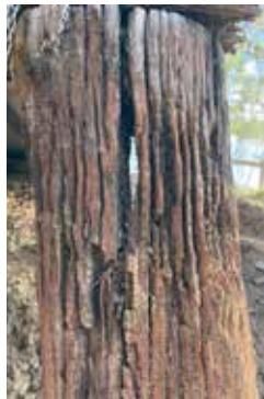
Part of the badly damaged pier.
